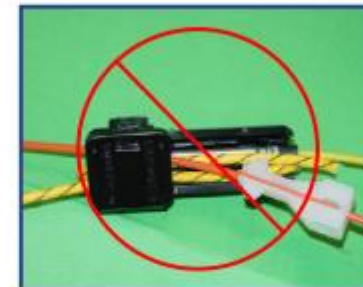
Figure 14 - Incorrect use of Bunch Block. Shock tube and detonating cord should NEVER be in the same block.
